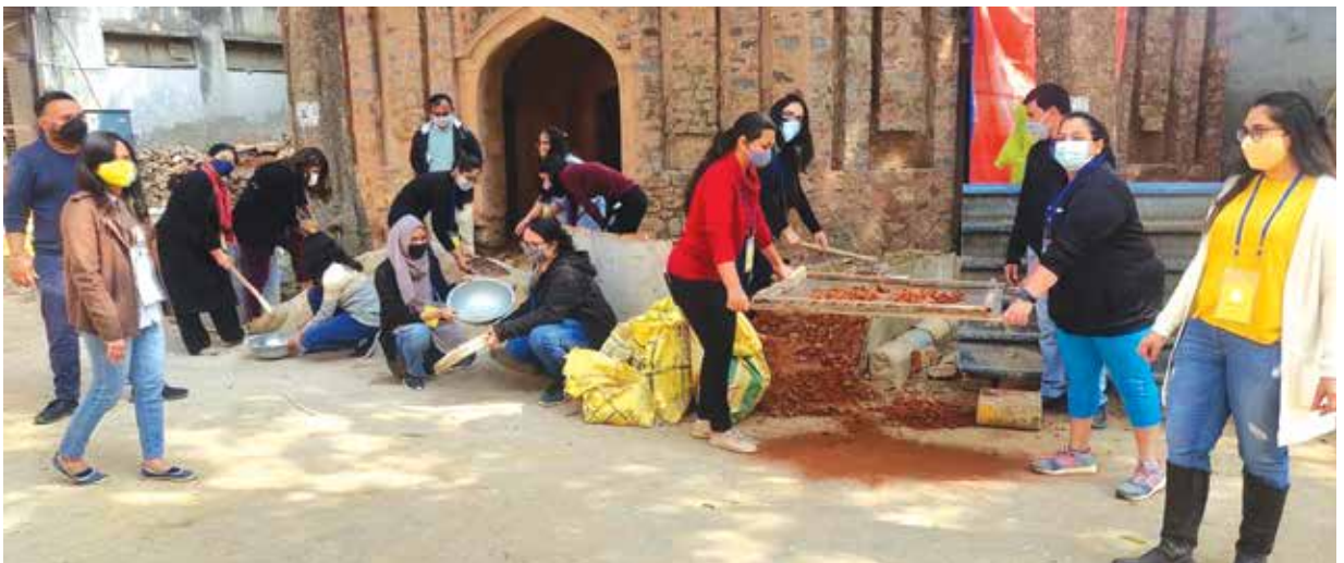
Students working at a site gaining practical hands on experience on Stone, Brick and Lime
